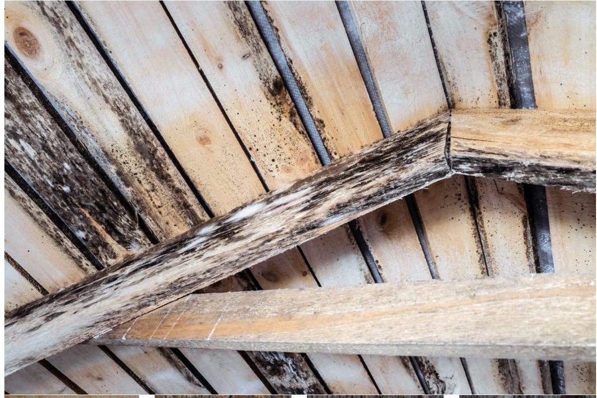
Severe mould infestation and irreparable damage to a roof structure
